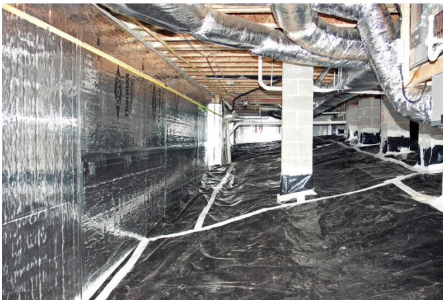
A tightly insulated attic in a home built by North Carolina's Eco Building Group helps keep the energy bills low.
